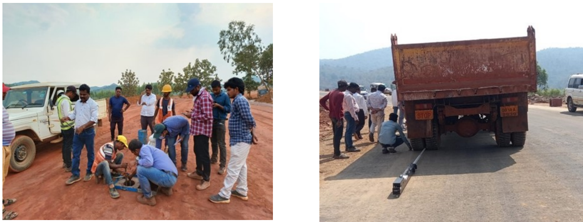
Figure 10. Field dry density test (left) and strength test (BBD) under progress (right).
